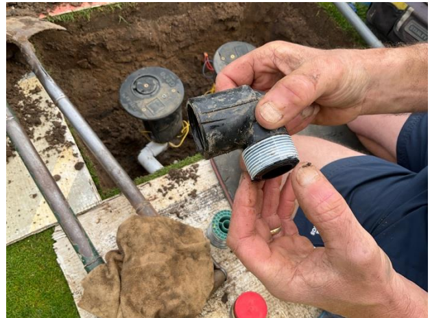
Photo 20: Problems have arisen due to the use of inappropriate connections on green side sprinkler pipework, which have subsequently failed.
