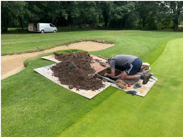
Photo 19: A reputable, outside irrigation contractor has been engaged to undertake key repairs on the sprinkler network.
