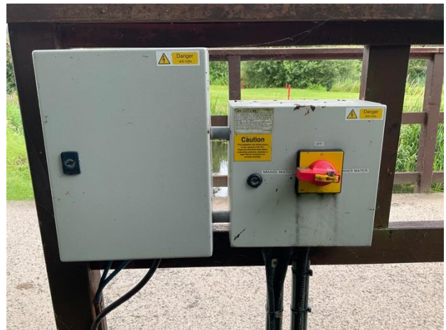
Photo 22: Switch controls, on the right of the above image, directs water supply from the river abstraction to mains when required.
